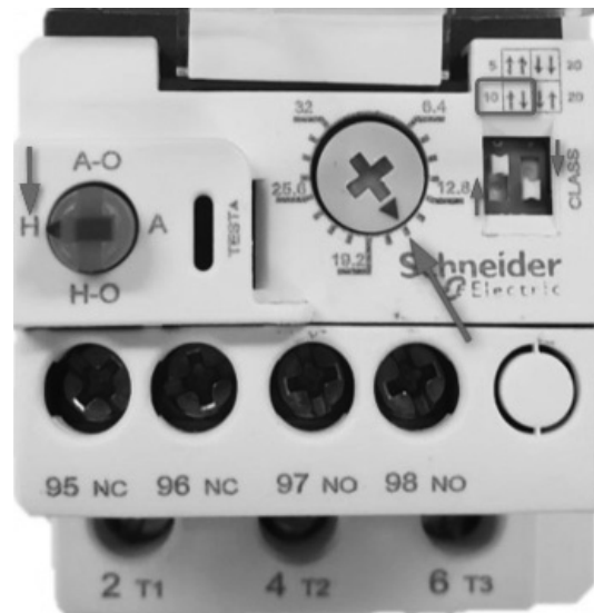
Figure 4 – 036-1 PSC & EON Units Overload Settings
